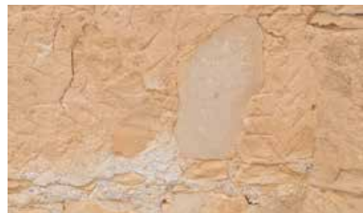
3.12. Plaster on the rear facade of the monument, with regular herringbone-patterned signs
