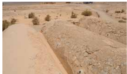
3.14. Exposed rubble core of the vaults' extrados, allowing water penetration and paintings' damage (before conservation)
